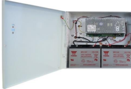
Figure 4 – Battery backup supply
