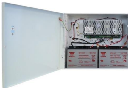
Figure 7 – Battery backup supply
