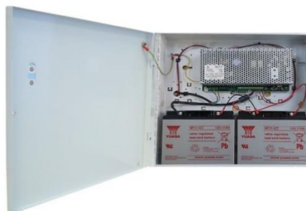
Figure 7 – Battery backup supply
