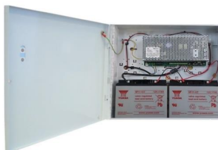
Figure 7 – Battery backup supply
